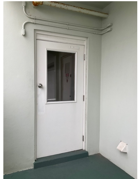
Unprotected glazed opening
