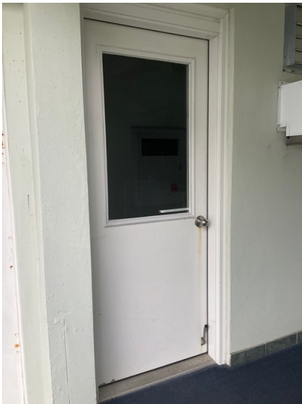
Unprotected glazed opening
