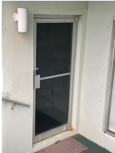
Unprotected glazed opening
