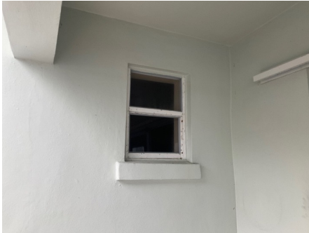
Unprotected glazed opening
