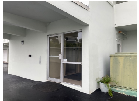
Unprotected glazed opening
