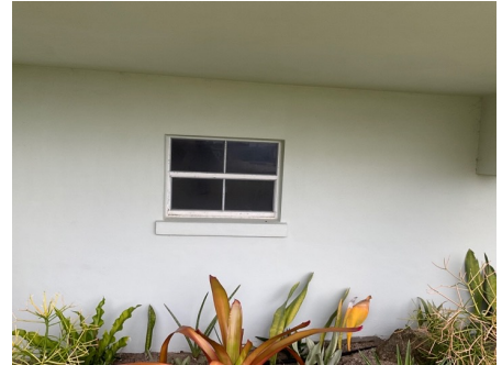
Unprotected glazed opening
