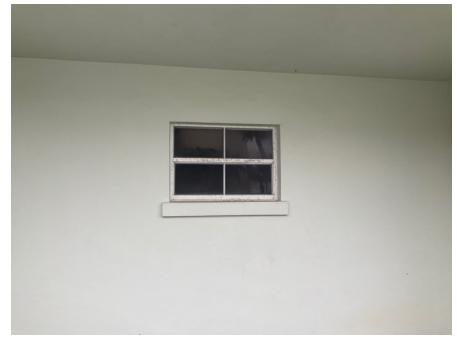
Unprotected glazed opening
