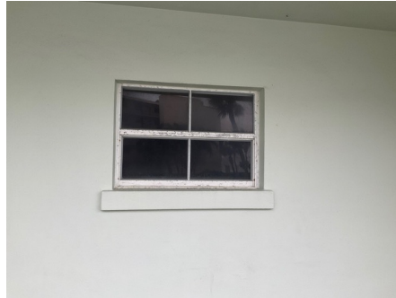
Unprotected glazed opening
