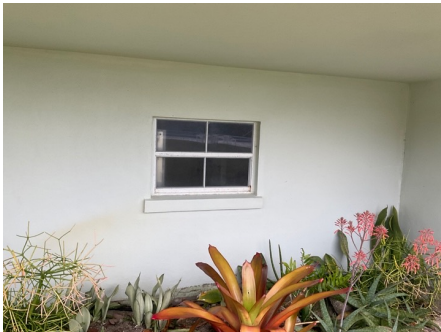
Unprotected glazed opening
