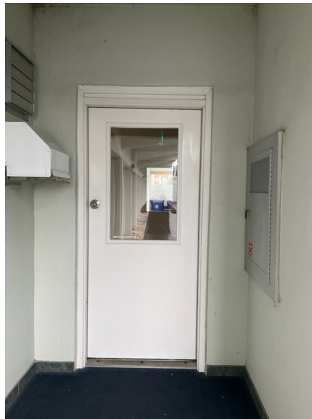
Unprotected glazed opening
